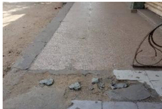
Figure (7) Unsuitable ground materials
